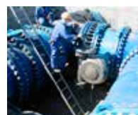
20 Shuweihat Water Transmission Scheme, Abu Dhabi, United Arab Emirates
